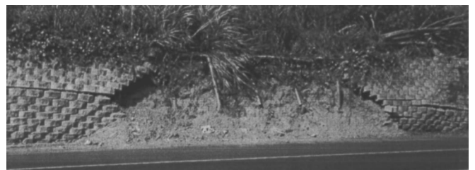
Fig. 2. Failure of modular-block reinforced-soil retaining wall (Ta Kung Wall)
